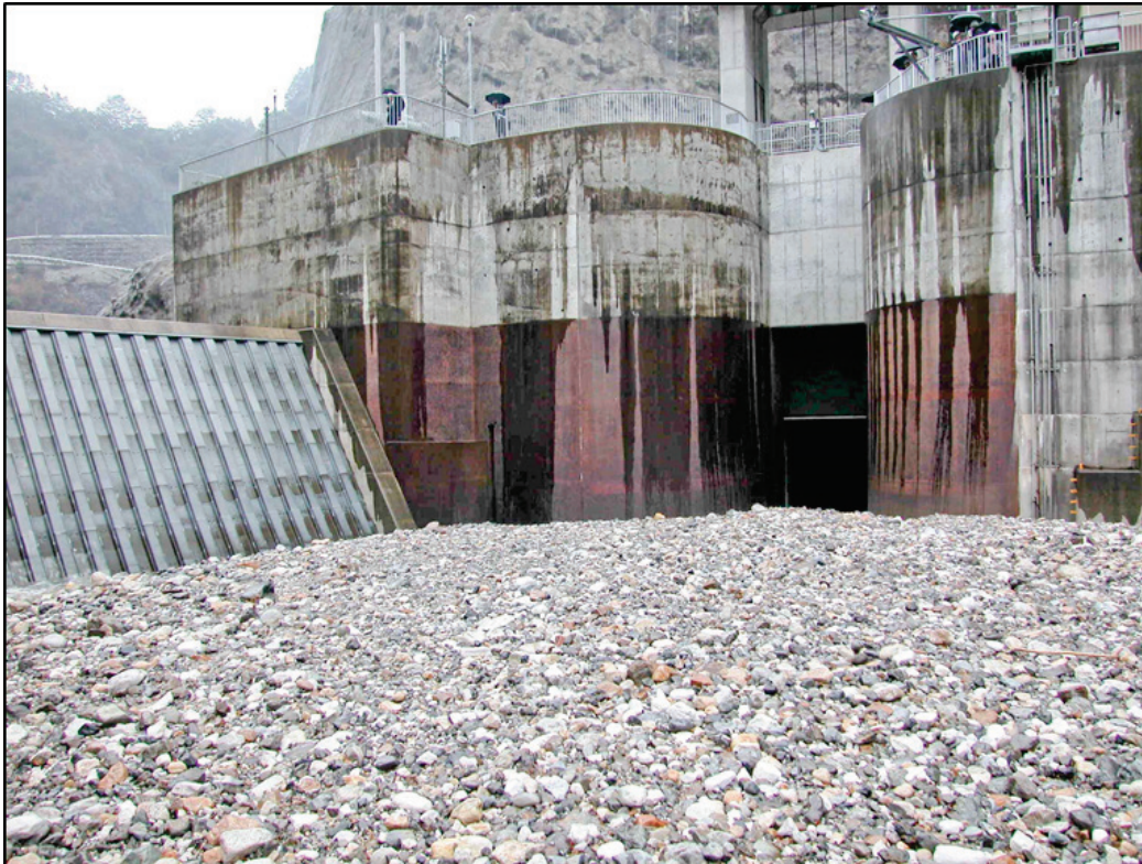
Figure 29. Upstream area of Asahi reservoir, Japan, shows entrance to gravel bypass tunnel on the right and cofferdam that directs flood flows into the tunnel entrance (photo G. Morris).
