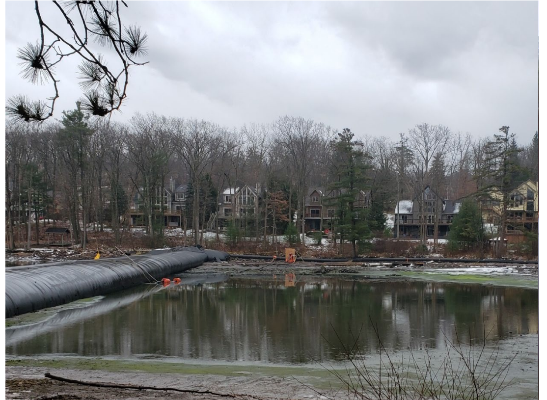
Water Bladder Dam
