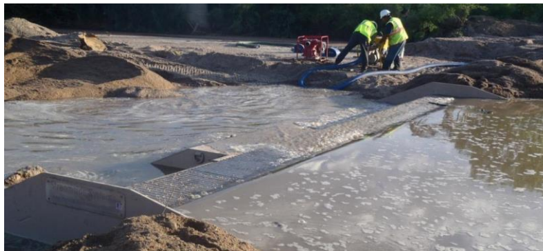
Figure 27 BI-T Collector Installed in Fountain Creek, Pueblo, Colorado, and Shore Sediment Re-Handling Plant
