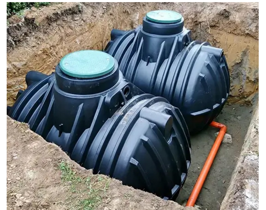
Underground water cisterns for larger scale rainwater harvesting Source LAIIEE; https://www.laiier.io/
