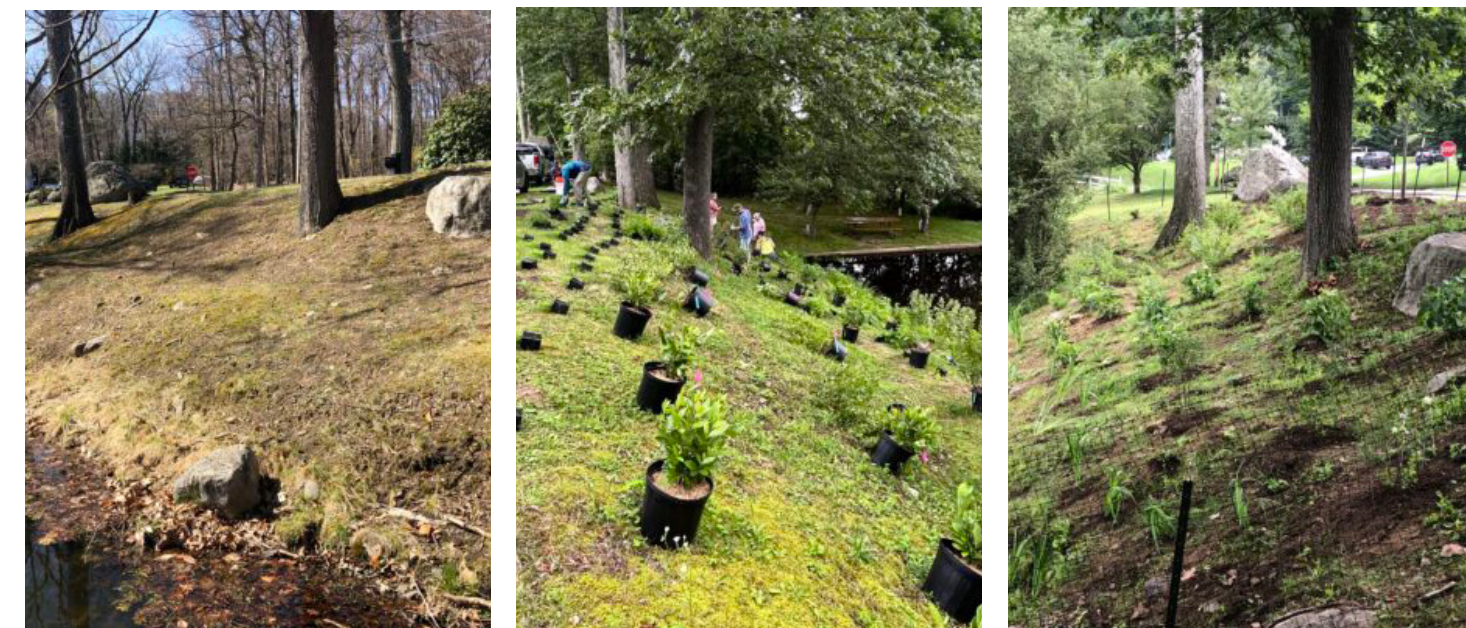
Before, during and after photos documenting riparian buffer installation; Designed by Princeton Hydro
